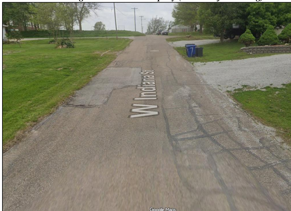
Road Leading to Mr. Weible's Property (2023 – Before Paving)
